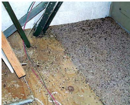
Figure 4. Heavy rodent contamination.
