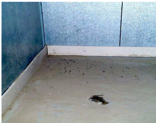
Figure 3. Light rodent contamination.
